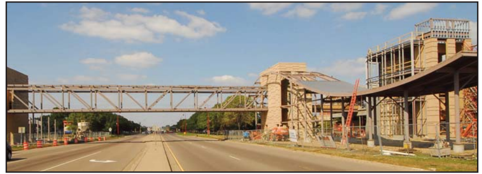
The Apple Valley Transit Station construction project is on schedule and on budget, with construction about 70 percent complete in late September, 2009.
