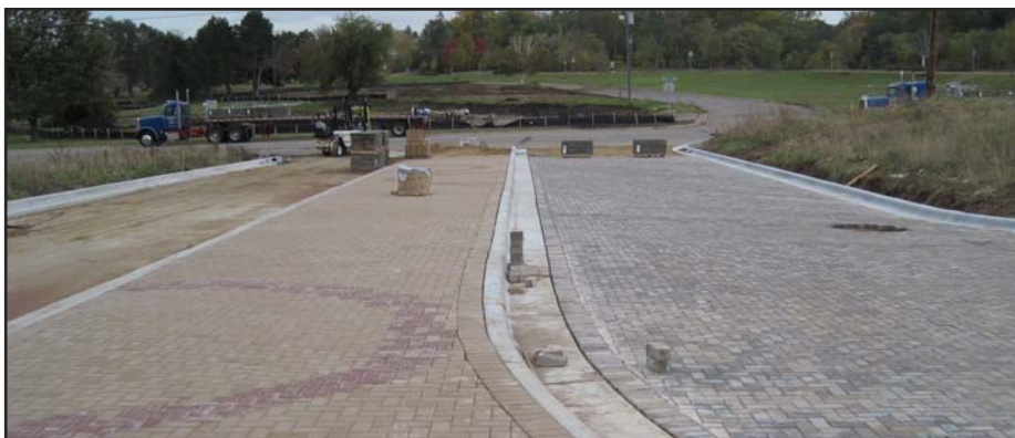
Pedestrians will be able to enjoy the patterned paver design nicknamed "Raindrops on Roses" due to the round "drops" of red pavers at the Cedar Grove Transit Station.
