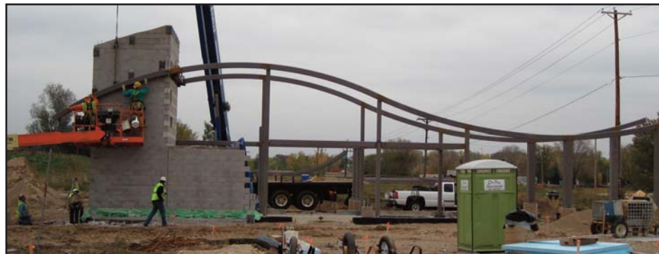
Construction is proceeding at the Cedar Grove Transit Station. Operations are expected to begin from this site in March 2010. More details will be included in future issues of the News That Travels . The site will support parking for 160 vehicles.
