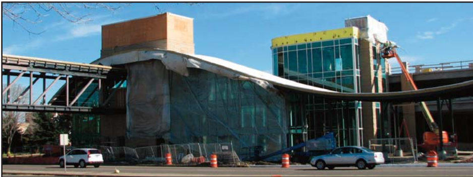
Watch for a special edition of News That Travels in December, featuring information about the opening of the New Apple Valley Transit Station. Service is expected to begin from the new site on Jan. 4, 2010 (check www.mvta.com for details). The site will support parking for 750 vehicles.
